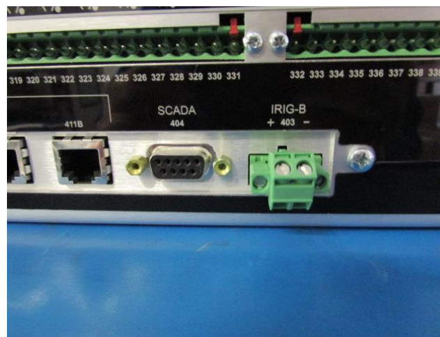
Figure 3. IRIG-B and SCADA RS-232 ports.
