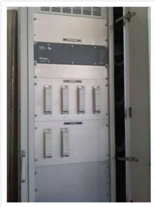
TESLA 3000 recorder installed in front panel.
