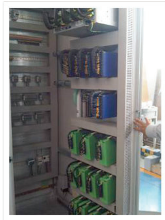
Back side of panel, showing PT/CT modules.
